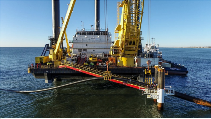
A support vessel for the horizontal directional drilling and cable-laying process for the South Fork Wind Farm ( Image: Michels, 2024 ).
